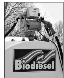
Biodiesel Fuel Tank
